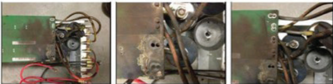
Figure 1. Capacitors with clear visual evidence of failure. Note, capacitors may fail with no obvious signs.
