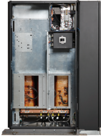
Front Access PDU with transformer access covers removed
